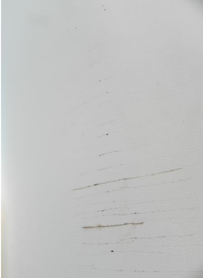
Figure 3. Parallel gel coat cracks.
